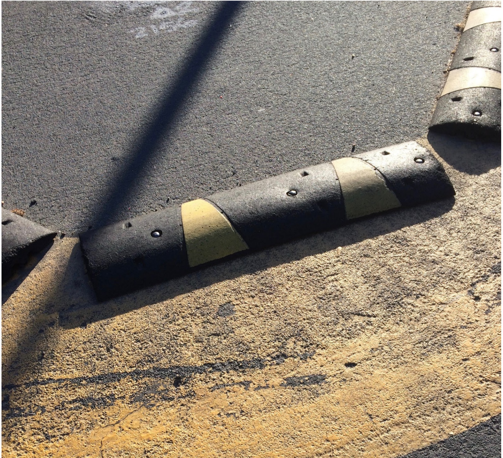
Detail of installation of speed bumps and paint to form traffic circle.
